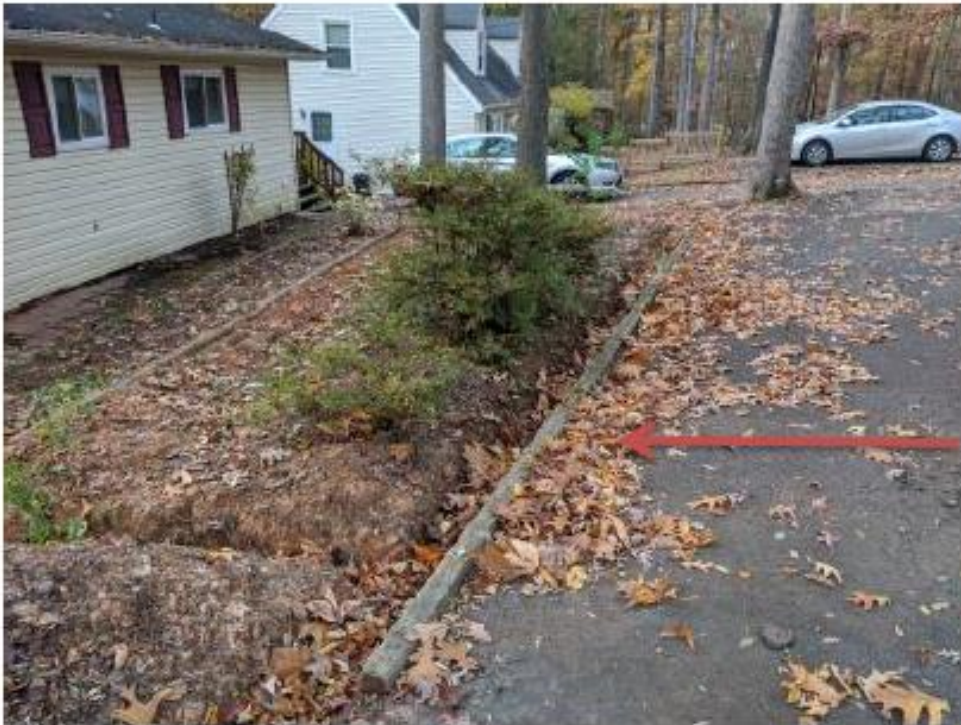
Driveway drains towards the house. Also shown is the partially completed excavation performed by a previous contractor.
