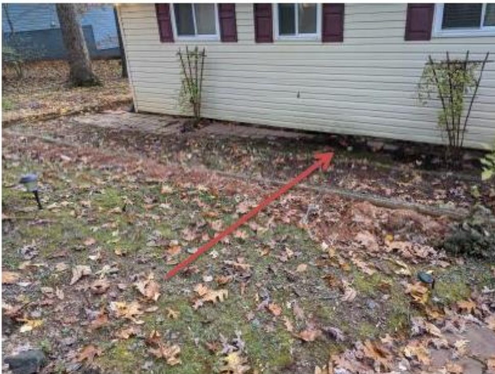
View of house foundation. Runoff from driveway ponds next to the house.
