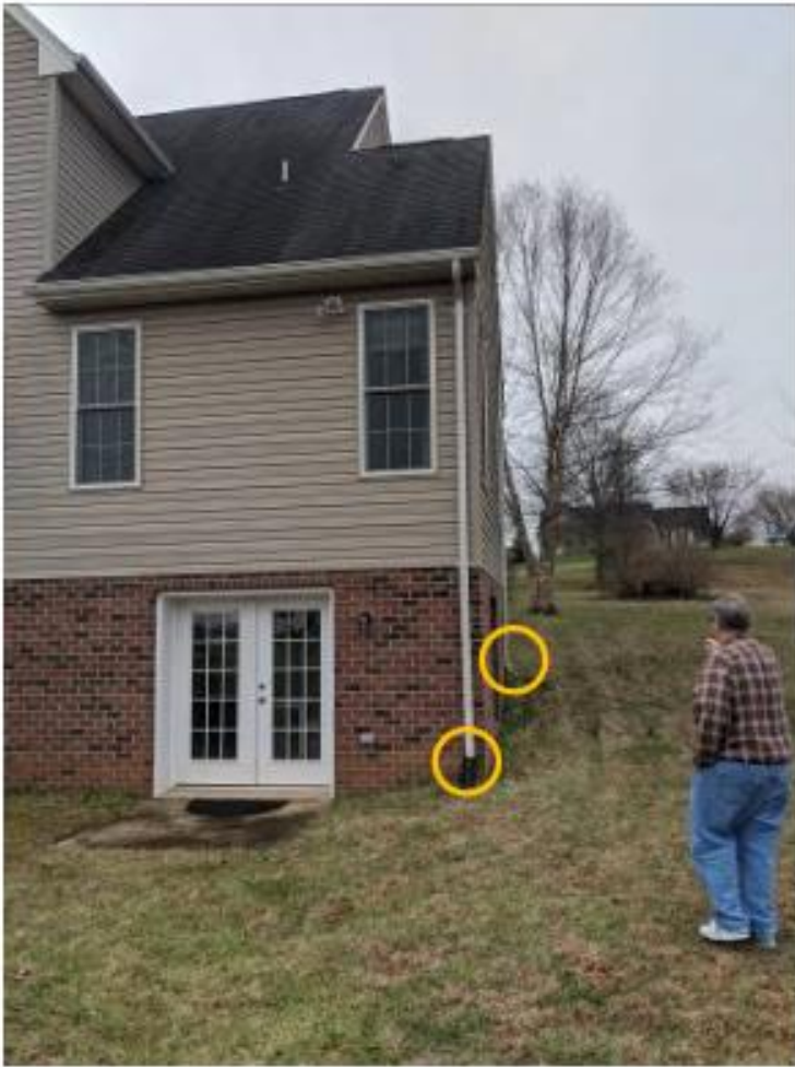
Downspout collection (#1 and #2)
