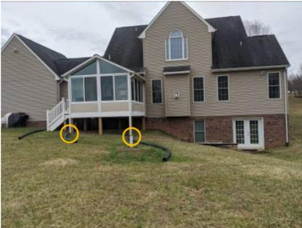
Downspout Collection (#3 and #4)
