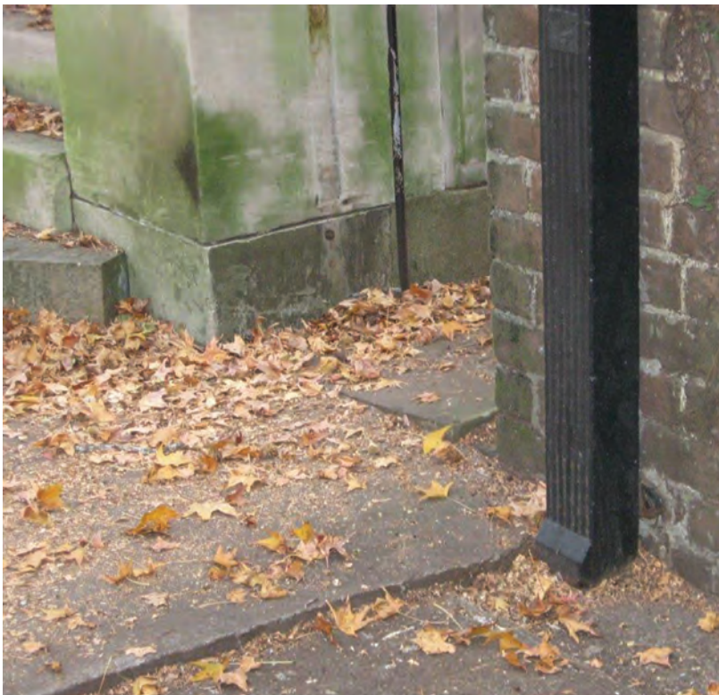
Figure I.4: Downspout piped directly to underground storm drain (Source: City of Savannah, GA).
