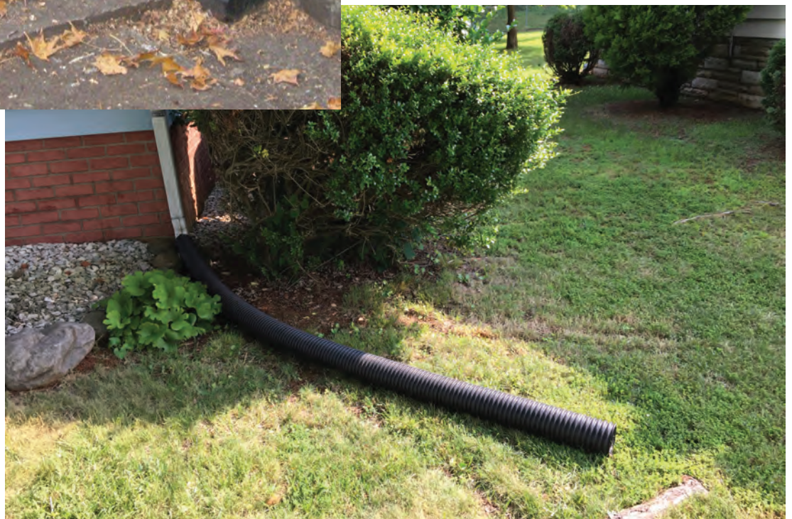
Disconnected downspout with extension pipe away from foundation (Source: Ted Millich)
